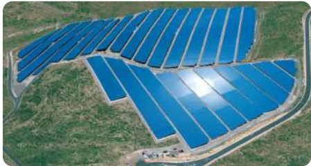
Enerife, Spain 13MWdc
